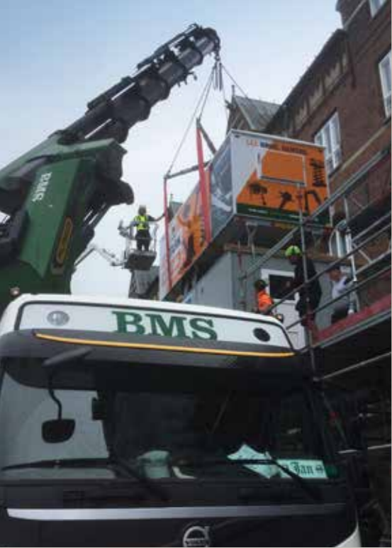
Placement of a pavilion on top of a similar structure at the City Hall Square in Copenhagen. The task was solved with a 165tm truck-mounted crane.
